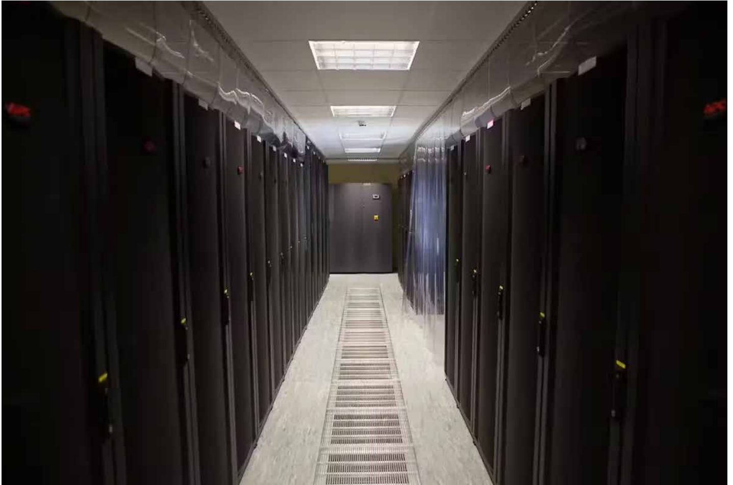
The server room at Cyberfort. PHOTOGRAPH: CYBERFORT/A.R.E. TAYLOR, CC BY
