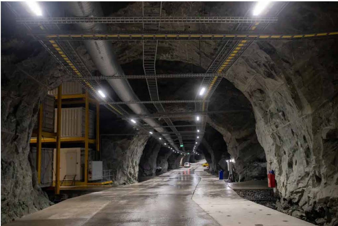
Underground: inside the Lefdal Mine Data Centers in Norway. PHOTOGRAPH: BLOOMBERG/GETTY IMAGES
